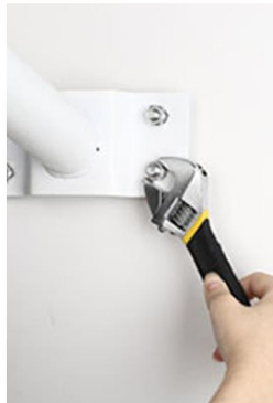
5. The installed light fixture is installed on the wall
